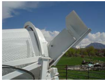
Figure 5 Chute gates are up to allow chute to close properly
